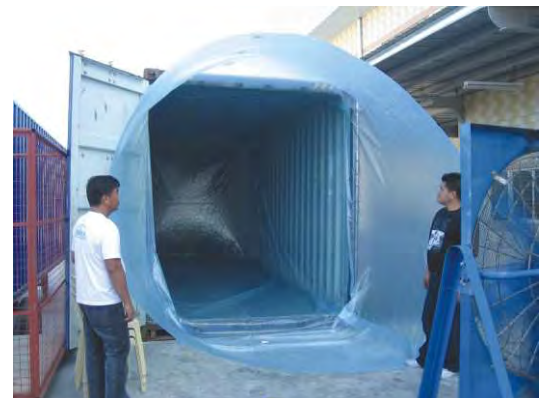
Installation of TSL using axial fan
